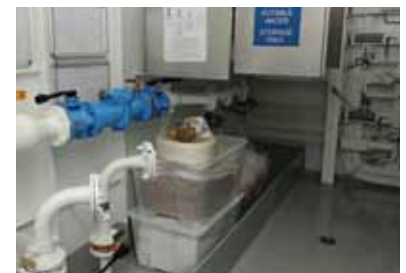
Potable water bunkering
