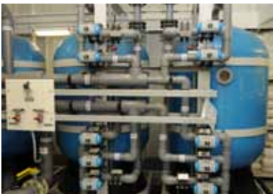
Reverse osmosis pre-filters
