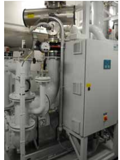
Components of the onboard Advanced Water Purification System (AWP)
