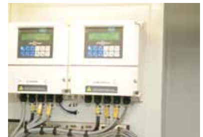
Potable water analyzer
